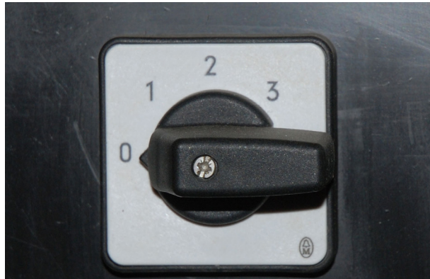
4-position switch for turning on the motors
