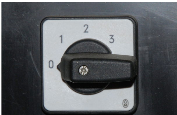
4-position switch for turning on the motors
